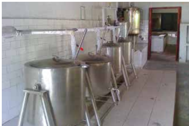
Picture 2: Steam cookers in use at the school's kitchen in Ladakh Source: Ladakh Renewable Energy Development Agency (LREDA)
